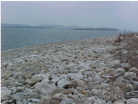
On site view of the 3.5 mile river levee riprap repair north of Lock & Dam 24 in Reach III.
